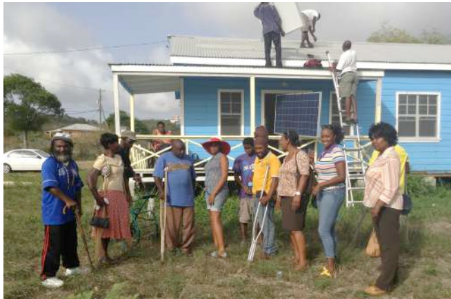
Installing the PV system at the Antigua and Barbuda Association of Persons with Disabilities
